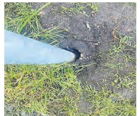
This photo shows that swings at the play area appear not to have been secured into the ground correctly.
